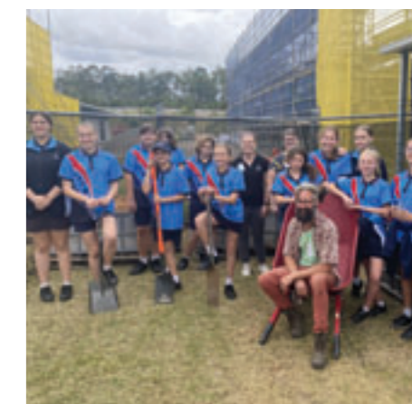
Yarrabilba State School in Queensland participating in a wicking bed workshop. They used their Lendlease Junior Landcare Grant to install water tanks and construct wicking garden beds to create a circular food economy.
